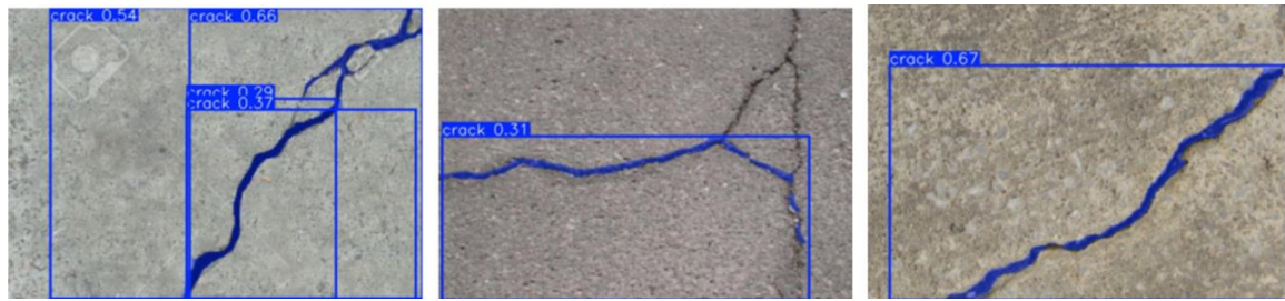
Figure 9. Result of Road Crack Detection
